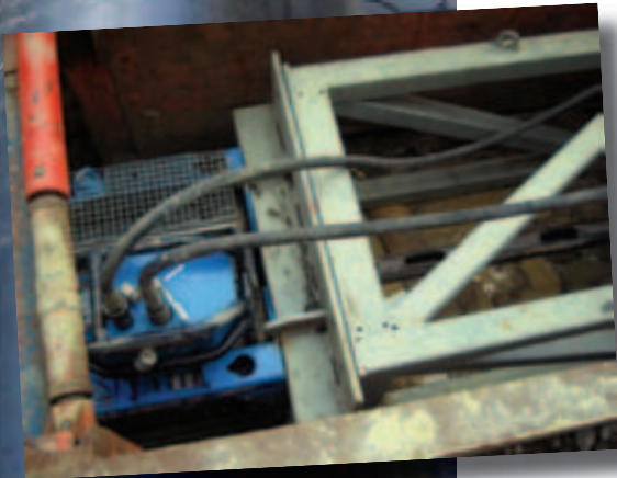
The Grundoburst 2500G rig with its extension frame in place during the Berlin swagelining operation
