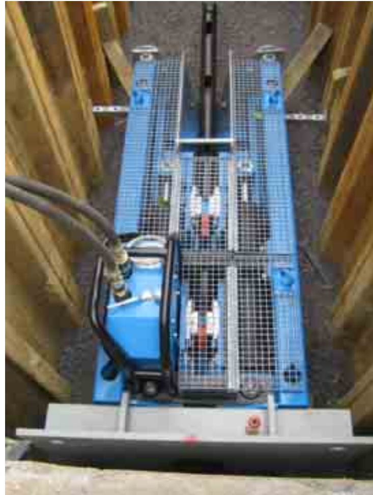
Grundoburst 2500 G in the machine pit.
