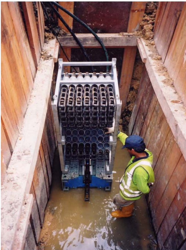
PHOTO 6: Shows the GRUNDOBURST 800G set up in the start trench where the patented Quicklock rods are pushed through the existing 4" AC pipe to be burst.
