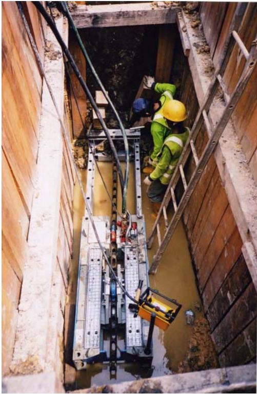
PHOTO 13 above – Shows the GRUNDOBURST 800G extended to allow the retrieval of the tooling and the 125mm PE pipe following the bursting operation
