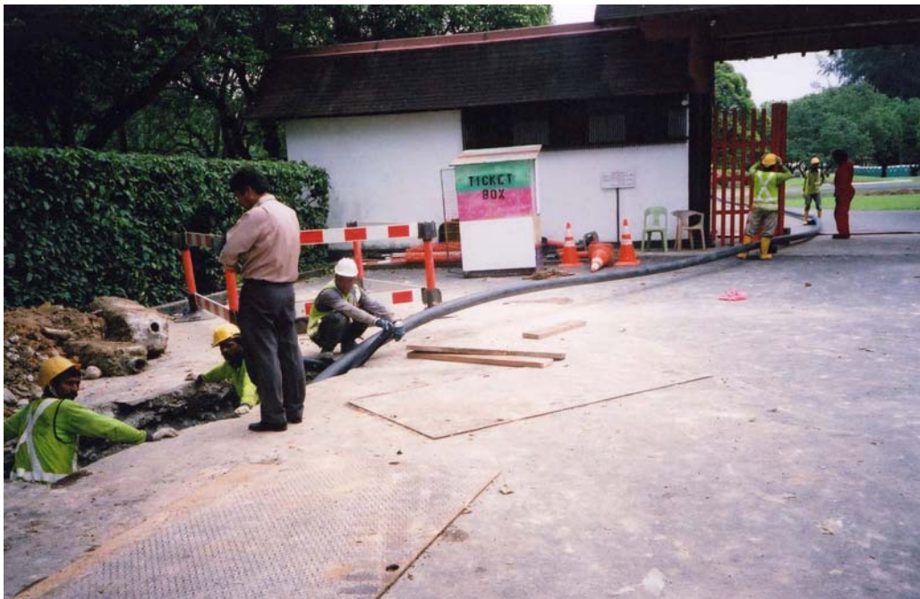
PHOTO 12 – Shows the 125mm PE pipe laid out during The bursting operation. Time taken to complete the bursting operation was 2 hours 10 minutes
